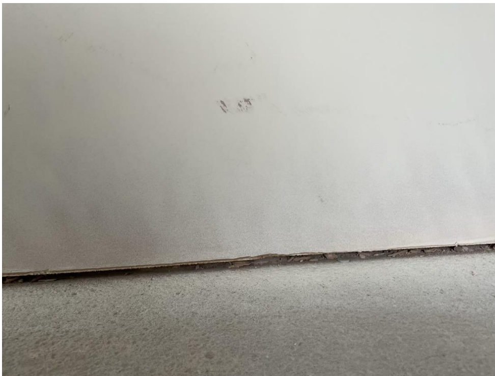
Photograph of drywall with board and plaster 10mm short of floor level (prior to filling).
