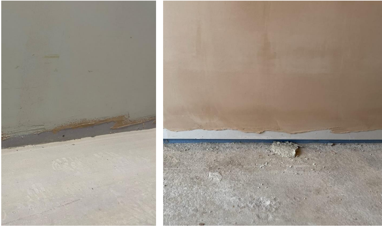
Photographs of drywall with plastering short of floor level prior to skirting application.
