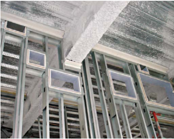
Figure 10 Prepared openings in a drylined partition (note spacings between openings may differ)
