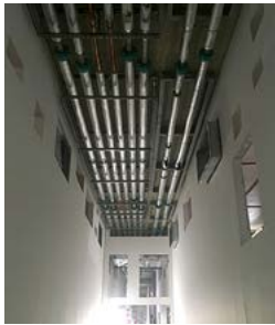
Figure 37 Penetrations created by dry lining contractor before services were installed
