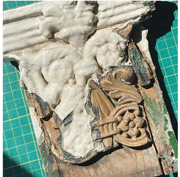
Figure 6: detailed composition ornament obscured under generations of paint from an external pilaster.
