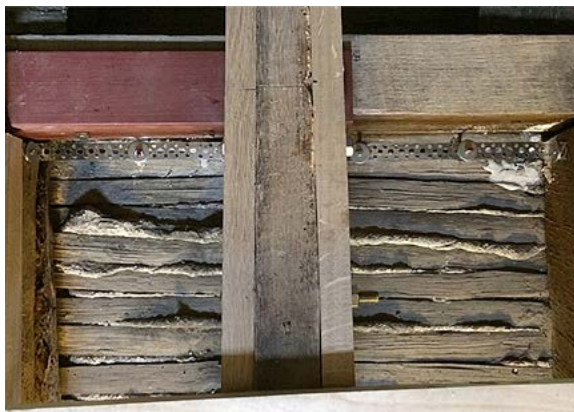
Figure 12. Low level steel strap and dowel suspending a delicate painted ceiling. Note the traces of grouting to the right.
