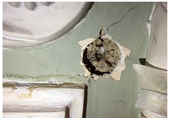
Figure 9: delaminated face coat and friable background, unsuitable for washer fixing, requiring both consolidation and grouting.
