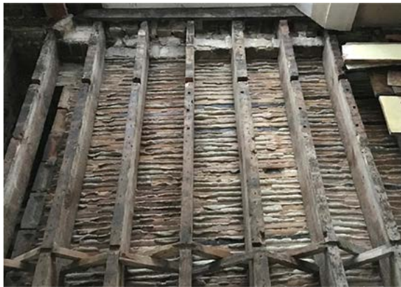
Figure 4: exposed ceiling void showing a good selection of nibs formed between laths.
