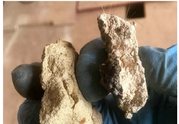
Figure 5: Georgian haired lime plaster (right), 20 th century lime gauged with gypsum (left).
