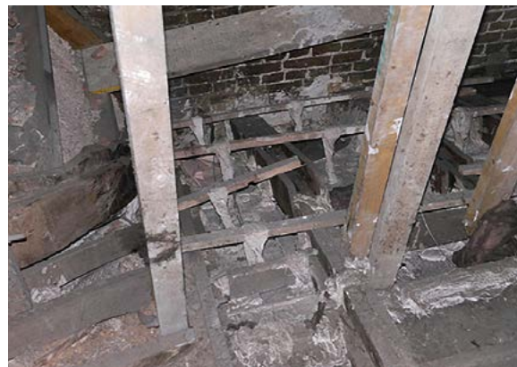
Figure 7: a Victorian church ceiling remains seen to the bottom, with areas replaced in fibrous plaster (middle) and expanded metal lath and hard, pink gypsum (left).
