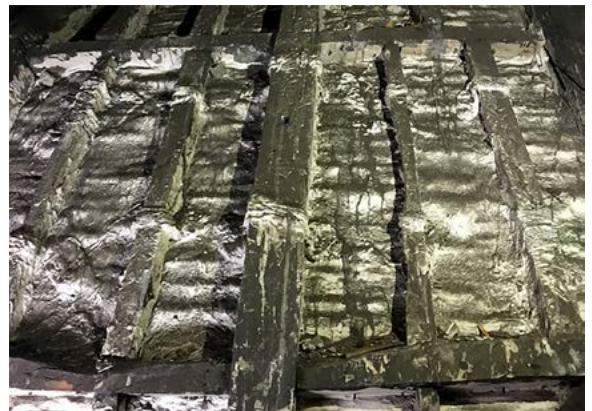
Figure 15: 1950s gypsum tray method to a dome post fire.
